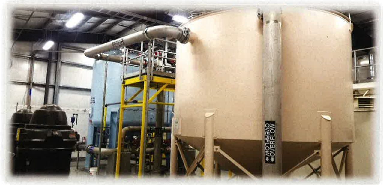
A Look Inside the Water Treatment Plant
